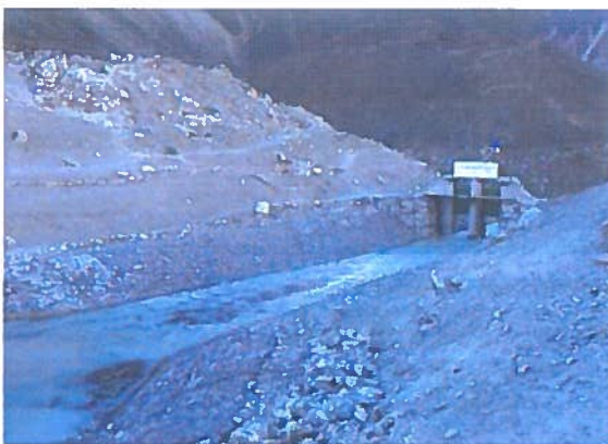
Figure 4: Open channel with regulatory gate constructed for draining the water volume from Imja Lake
