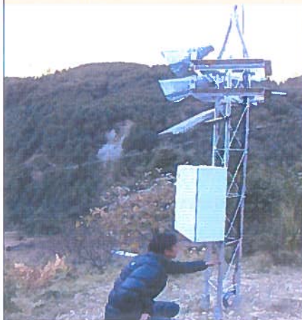
Figure 2: Nawang checking the automated Siren installed in Phakding
